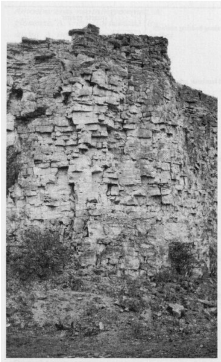
(Figure 4.36) View of the northern face at Leysthorpe Quarry, showing the thick Malton Oolite sequence, with, at the top, a thin development of Coral Rag overlain by thin-bedded, flaggy Upper Calcareous Grit. (Photo: J.K. Wright.)
