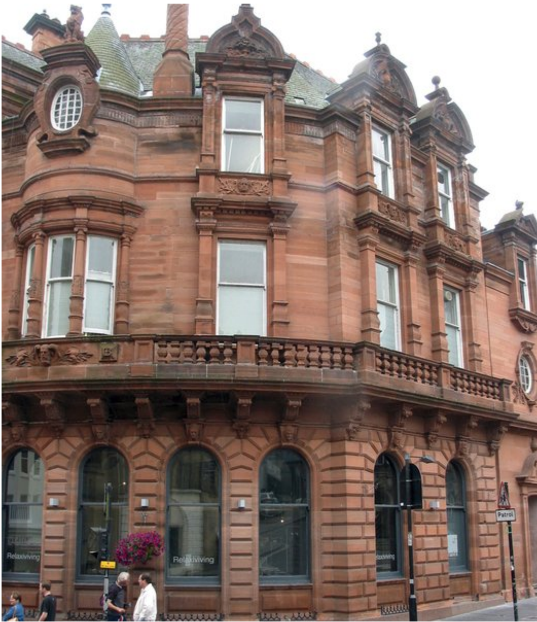
(Plate 1.2) Locality 1.10. 61 King Street, former Clydesdale Bank; red Permian sandstone from Locharbriggs.
