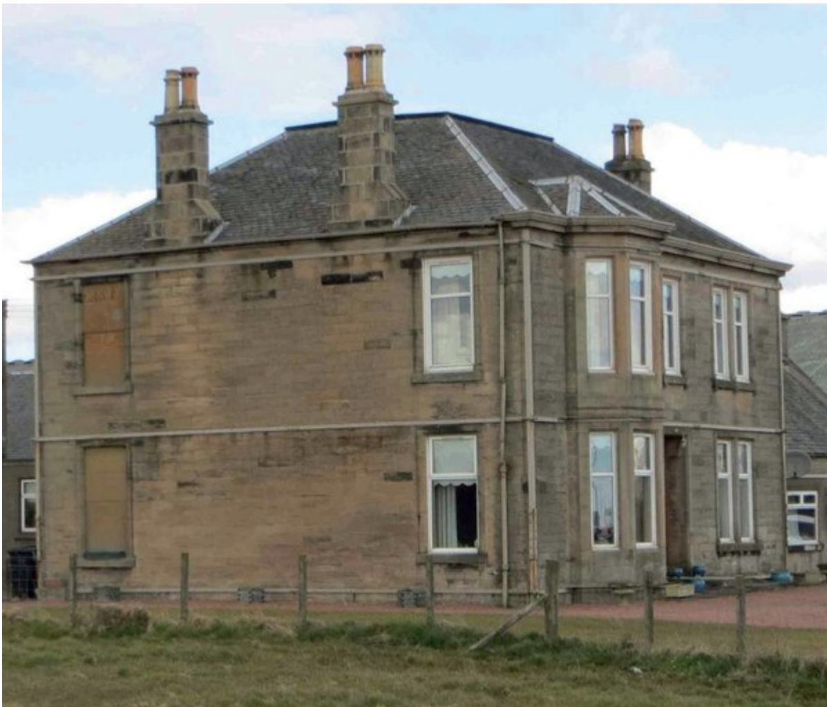
(Plate 3.3) Locality 3.4. Evidence of ground instability due to shallow coal workings; house with restraining horizontal and vertical metal straps, near Bellsdyke roundabout.
