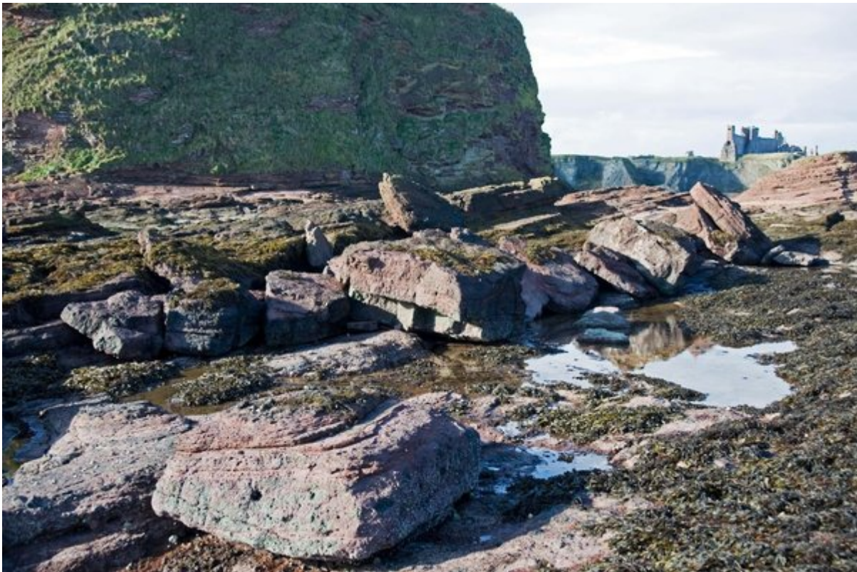
(ELC_25_P3) Undercut collapsed blocks on the shore platform at The Gegan. © John Gordon.
