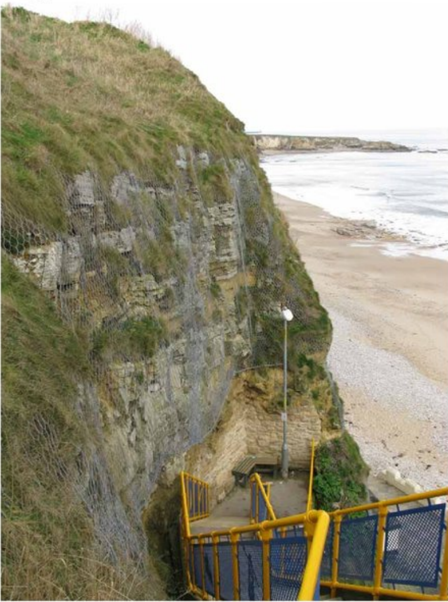
(Plate 13) Wire mesh protection of the cliffs near the steps at Marsden Bay. The nature of the rocks can still be seen through the stabilisation measures (February 2009).
