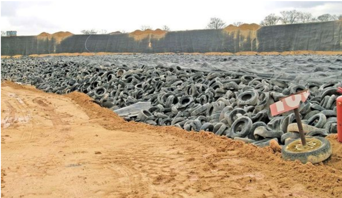
(Figure 42) Tyres from Hampole Lime Works Quarry used as drainage layer. [SE 49950 11050].
