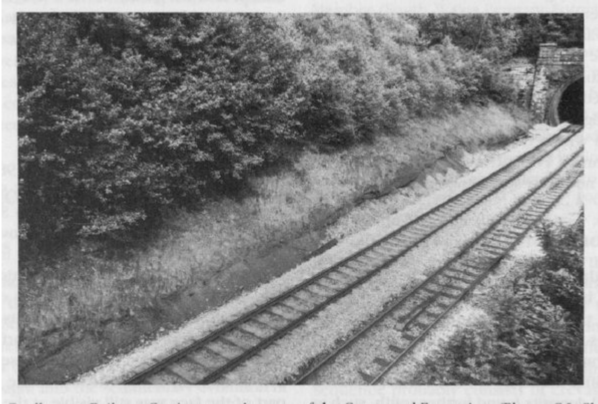
(Figure 4.25) Penllergaer Railway Cutting exposing part of the Grovesend Formation. (Photo: C.J. Cleal.)
